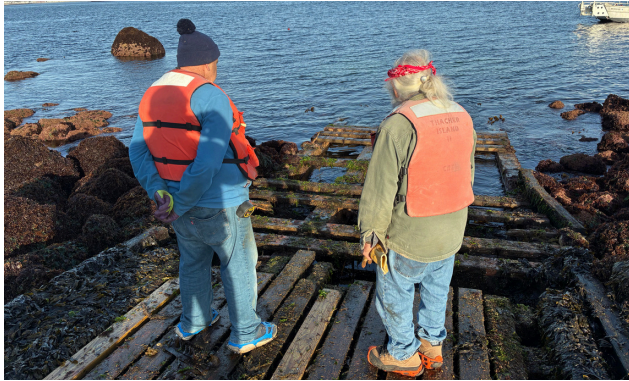
Paul Sena and Doc Wedmore inspect the decayed end of the Thacher boat ramp. Photo credit: Bill Whiting
