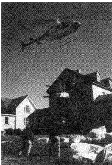
Helicopter drops a load of shingles for the roofers and picks up bags of old shingles for disposal.
