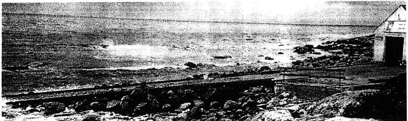
Finished ramp looking north, note the 4-5 ton riprap boulders protecting the edge of the ramp on both sides.
