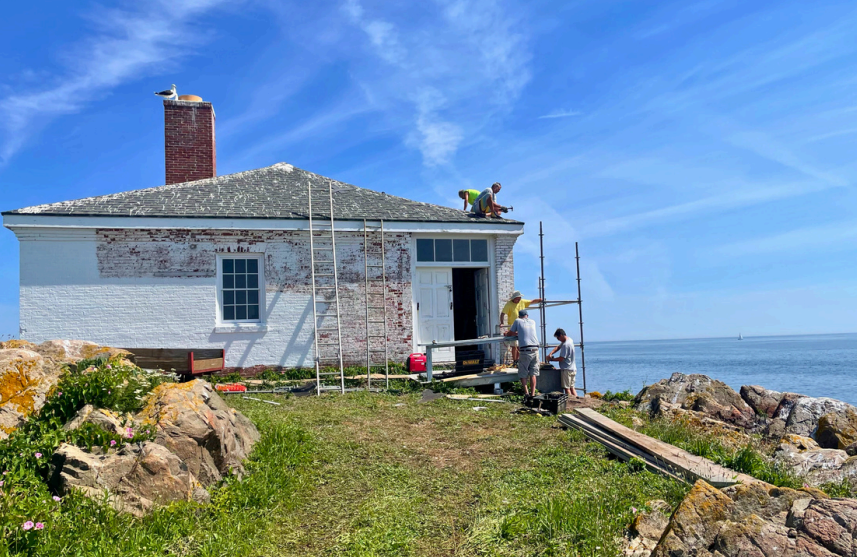
On Whistle House: Jon Conant and Joe Napolitano repair the roof; Bill Sclafani, Bill Whiting, and Mike Hammerl erect scaffolding to repair the east wall.
