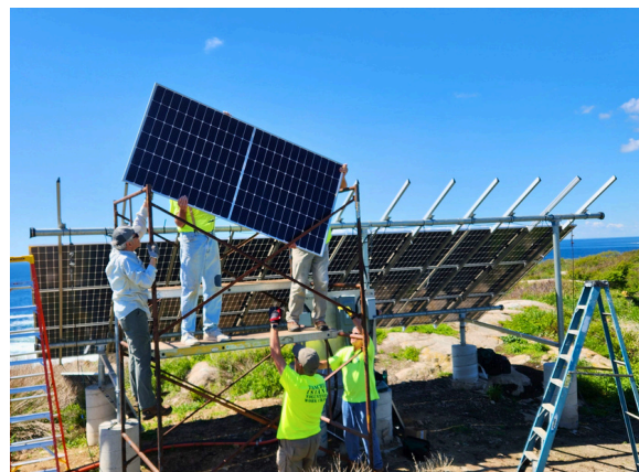
Tom Mikus, Ray Moss and Dave Anderson (hidden), Bill Helmuth, and Dick MacPherson install the last row of new solar panels on Thatcher.
