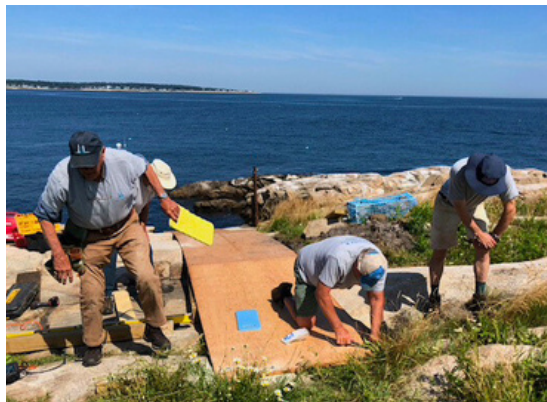
Peter Bergholtz, Dave Anderson, and Nathan Ives construct temporary ramp for delivering materials.
