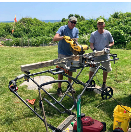
Bill Whiting and Bill Sclafani build housing for the generator on Straitsmouth.
