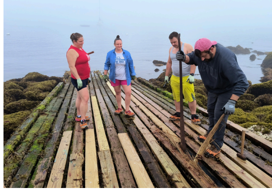
Sarah Glick, Dorothy Maglione, Dan Kosinski, and Tony Maglione replace rotten planks on the Thatcher Boat Ramp.
