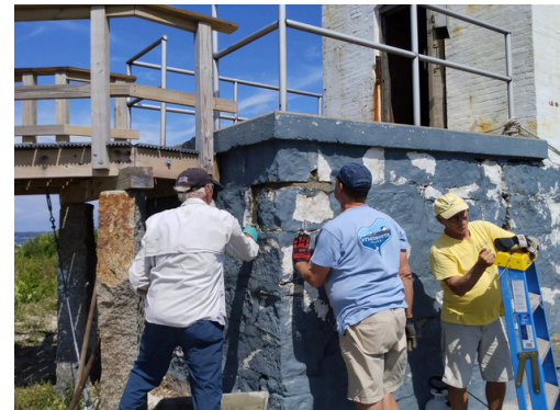
Peter Chick, Randy Saville, and Bill Sclafani scrape, repoint, and paint Lighthouse base.
