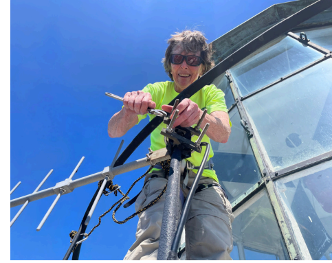
Donna Cusick removes an unused antenna from the Thatcher South Tower parapet to allow replacement of the railing.
