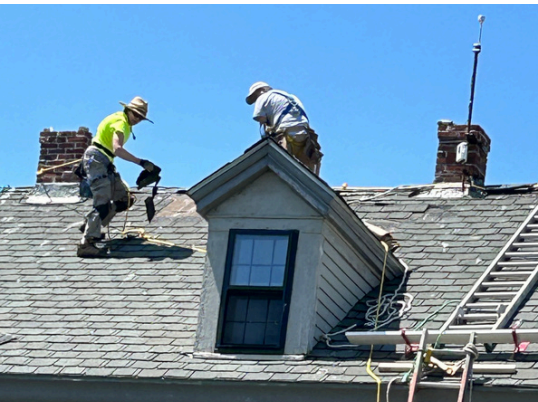
Donna Cusick and Fred Stoddard repair winter damage to Thacher Assistant Keeper House roof.
