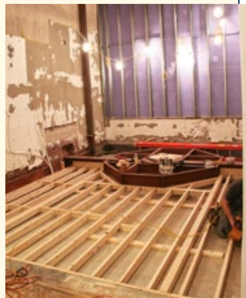
Steel base installation. Gallery sub floor installed around special steel support girders. Photo courtesy of Leon Doucette, Cape Ann Museum.
