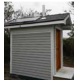
Solar panel and siding.
